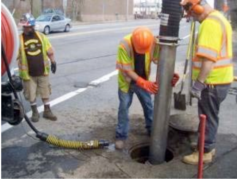
COURTESY URI TRANSPORTATION CENTER CLEAN WATER: R.I. Department of Transportation workers clean a storm drain using a vacuum pump and a vehicle called a "vactor."
